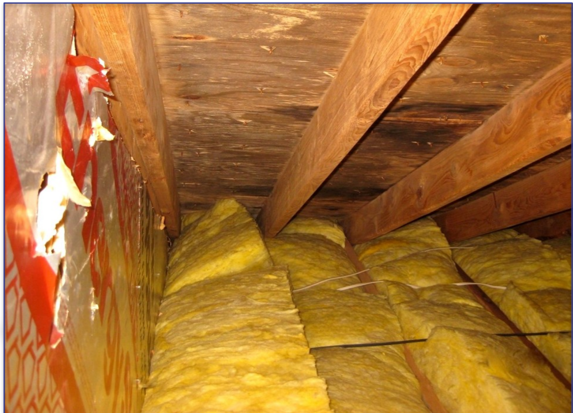
INSULATION OVER SOFFIT OR LACK OF INSULATION
